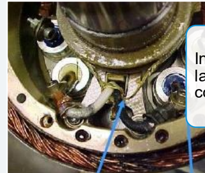
Defect in design
